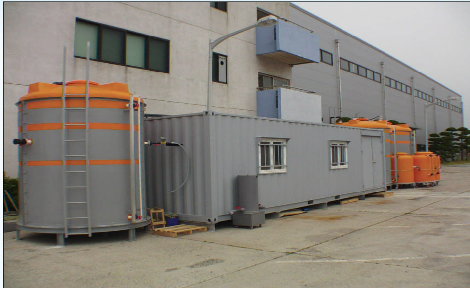
Pilot plant (5 m 3 /hr)
